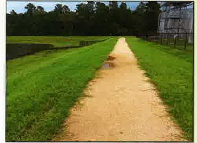
Top dressing of 1"-2" of granite to fill low depressions, crown to drain.
