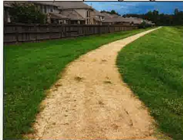
Portions of trail have visible signs of geo-fabric visible. repair trail to 5" depth .
