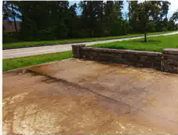
Maintenance access not utilized -Possible seating amenity.
