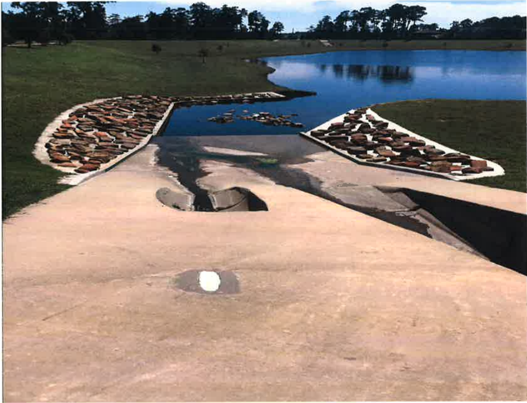
Armored slopes at the inlet from storm drainage system held up very well
