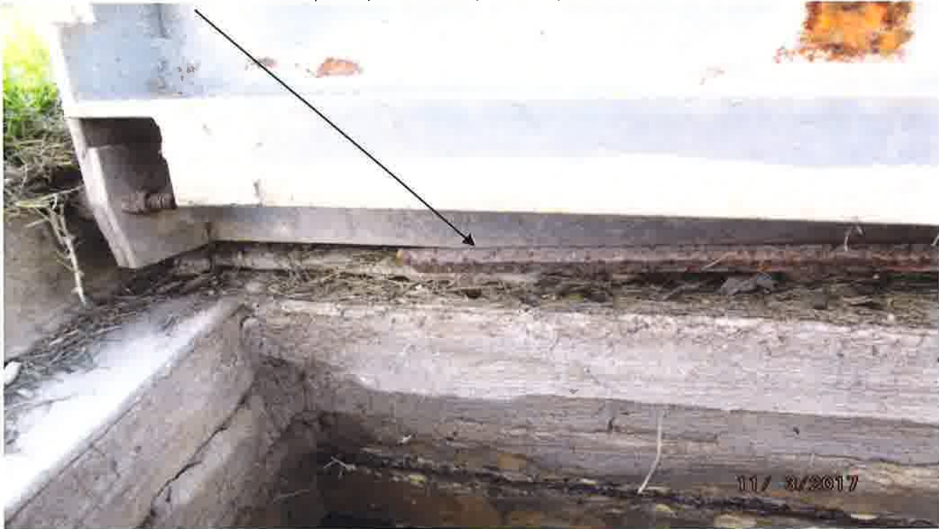
Broken torsion bar on the entry door presents safety issue for personnel entering and leaving the unit.
