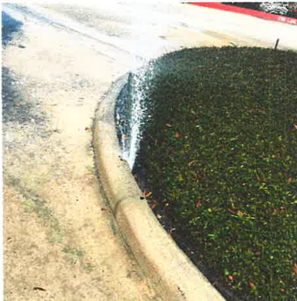
Zone #14 (Valve Status) - 03-18-19 3:11 pm CDT
